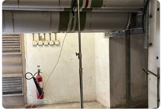
Tripod / mast camera — deployed in a plant room in minutes.
